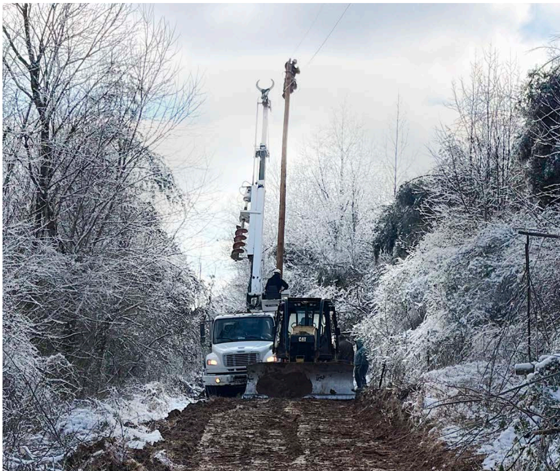
▶ Fleming-Mason Energy Lineman Josh Hamm climbs a pole while working mutual aid for Tri-County Electric. Photo: Tri-County Electric Foreman Steve Emmert
